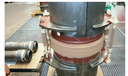
All stainless steel components and drill holes are masked for the multi-layer coating of the carbon steel parts
