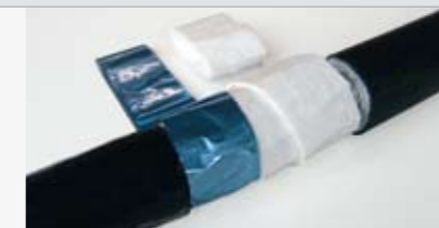
Wrap the self-adhesive glass-fibre tape around the hose and the fitting only. Then wrap the heat-reflective, self-adhesive tape, allowing a 25% overlap.
