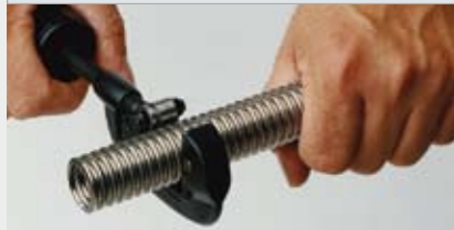
Cut hose to the desired length in a groove of a corrugation using a pipe cutter.
